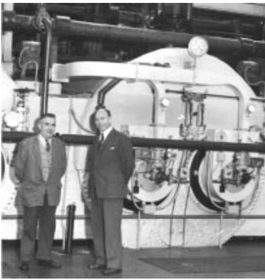
Jack Stimpson and James Salmon by the boilers (newly converted from coal to oil) in 1961
